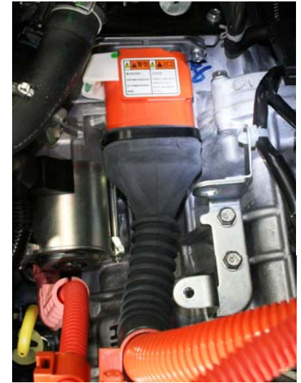
High-Voltage Cable Connection to Motor
